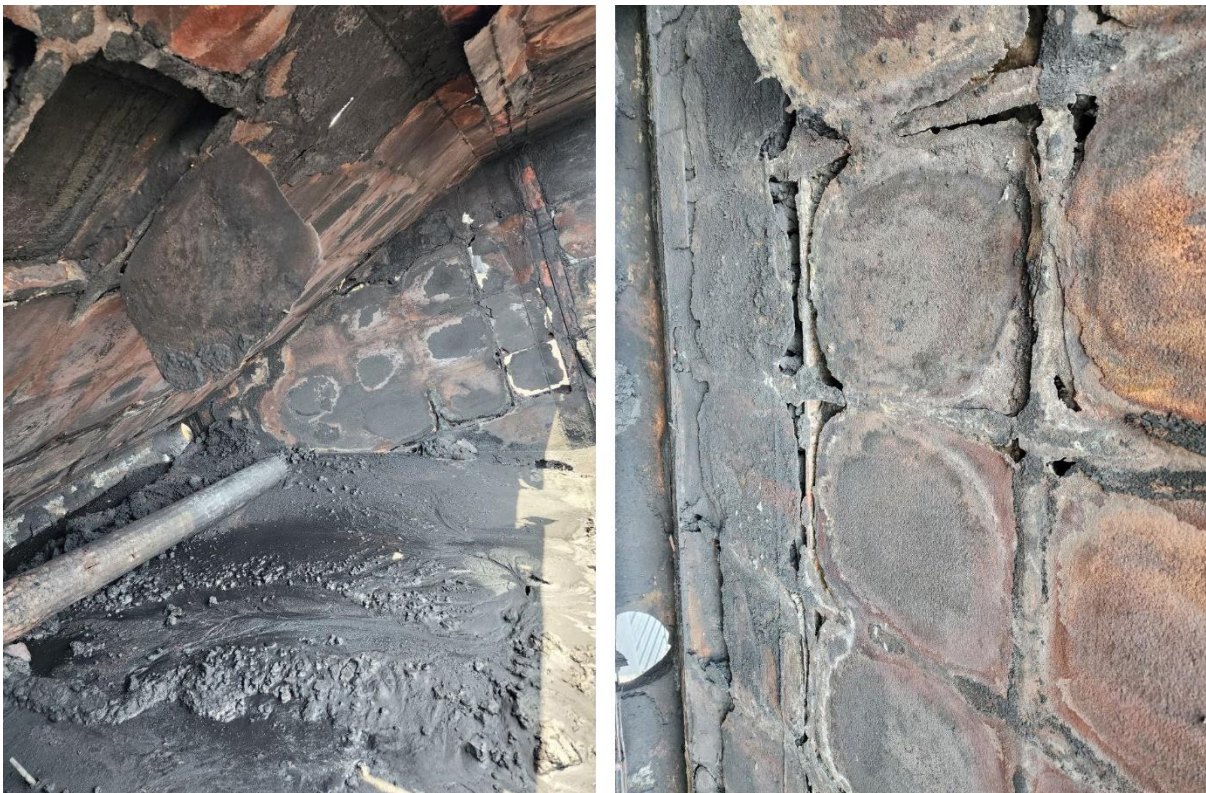
Fig. 1. Failed exhaust bag filter with severe corrosion.
